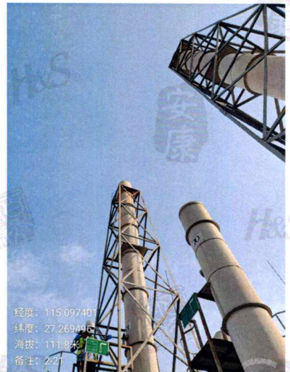
2-21#外层蚀刻线(蚀刻段)废气排放口
