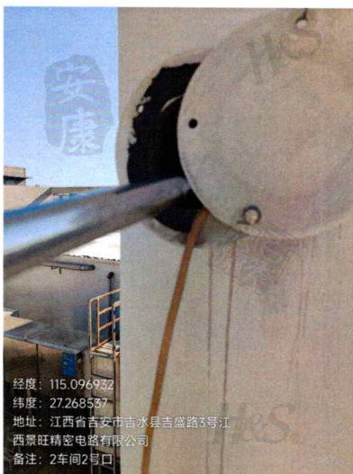
2-2#内层涂布有机废气排放口
