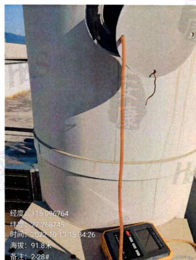
2-28#防焊预烤废气排放口
